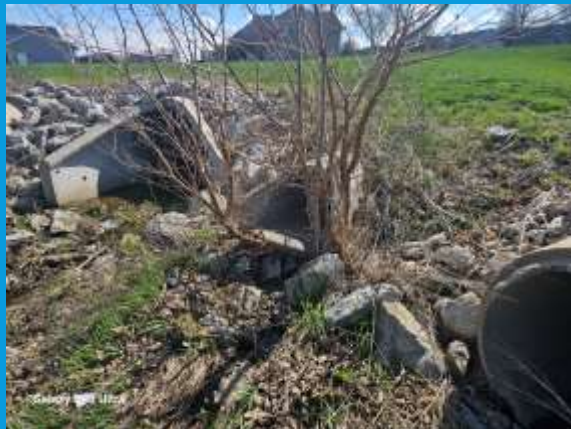
Trees blocking culvert
