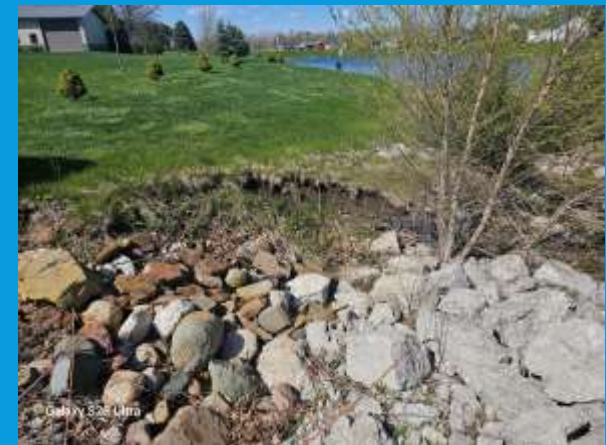
Washout along west side
